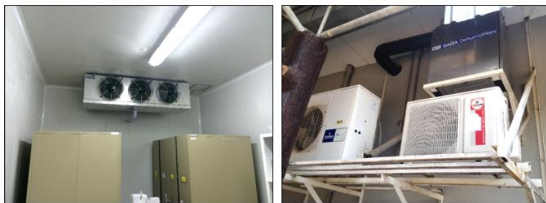
Figure 8 Refrigeration and Dehumidify system of Seed lab
